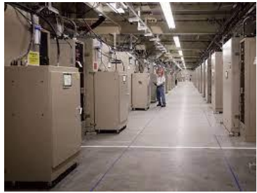
Capacitor banks (~400 MJ)
